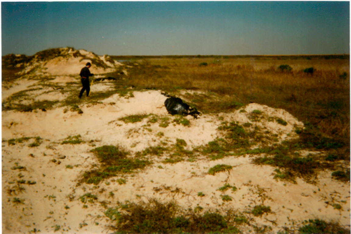
Photograph No. 2. View to the southwest showing an eroded section of the south berm and the damaged polyethylene liner.
