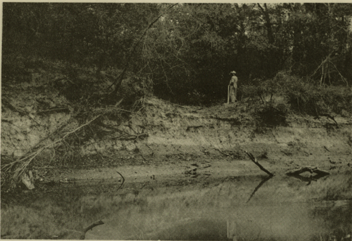
Photograph 4 View of notch in right bank at A. Cut into gray silty clay. Sand at top of bank and near water edge.
