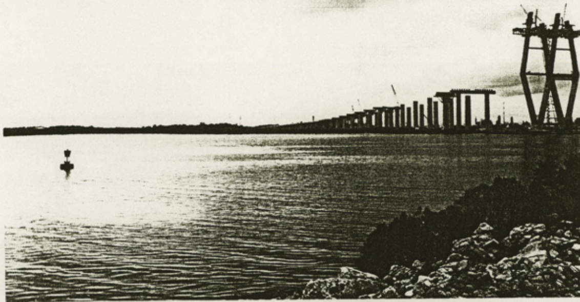
Looking southwesterly across the Houston Ship Channel at the northern end of Spillman Island where Highway 146 crosses the subject property.
