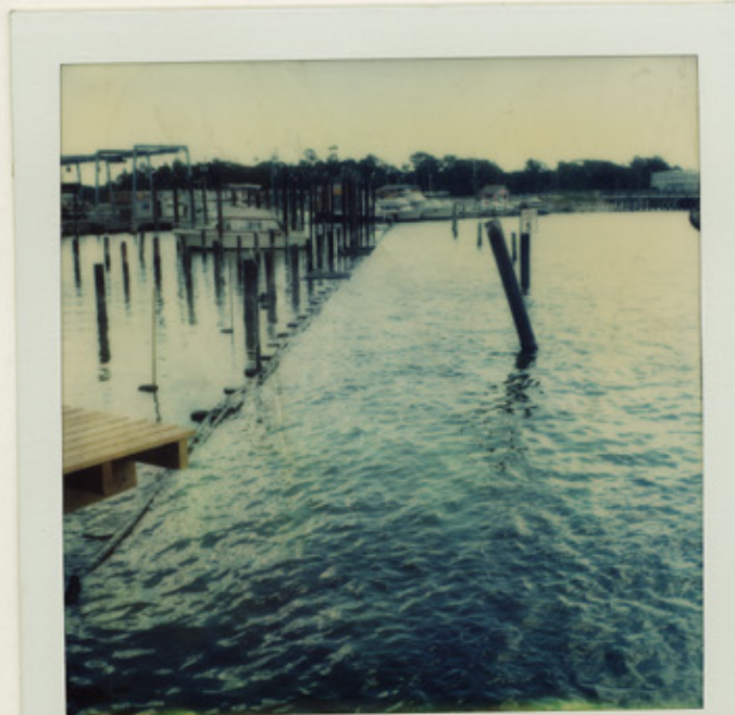
Photo #2 - Standing on new structure looking toward Nasa Rd. I at old bulk- head with pilings in front
