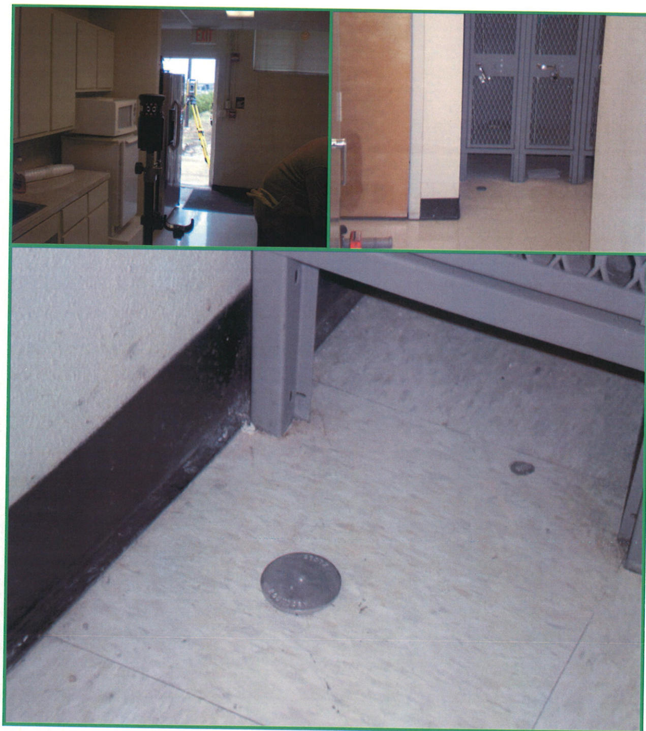
Fig. 8. Above left: Traversing into the south side of Building 41. Above right: Location of the Camp Mabry boundary monument 2.4 feet inside the outer wall of Building 41. Below: 5/8" iron rod with aluminum cap stamped AGDTX-BOUNDARY set for corner.
