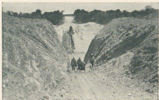
Cutting down through the banks of the Arroyo Colorado to lay the big mains for natural gas supply which is one of the greatest assets the Valley has.
