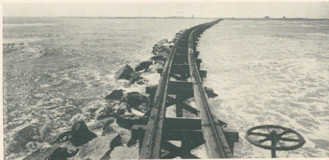
The United States Government has built jetties at Point Isabel and is in charge of harbor work there. A sixteen-foot channel is already dredged, and the Valley expects to get a thirty-foot channel by creating a navigation district, and through Government aid.
