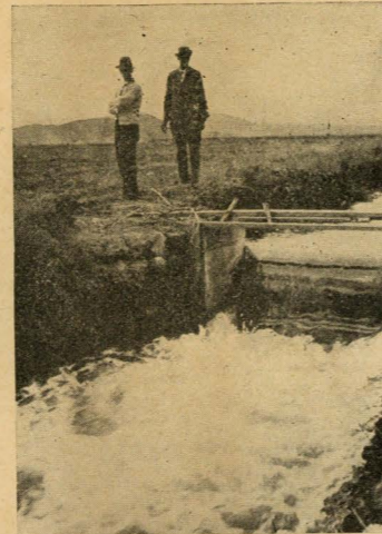
Irrigation Service Canal in the Pecos Valley
